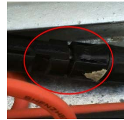
The cable is loose
